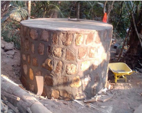
a) 10 M3 water tank
